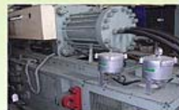
2 nos Kleenoil 9788 hydraulic units installed on an injection moulding machine
